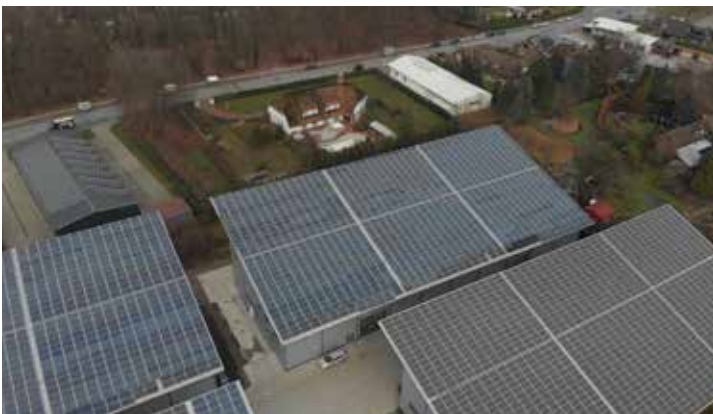
Solar panels that power the facility
