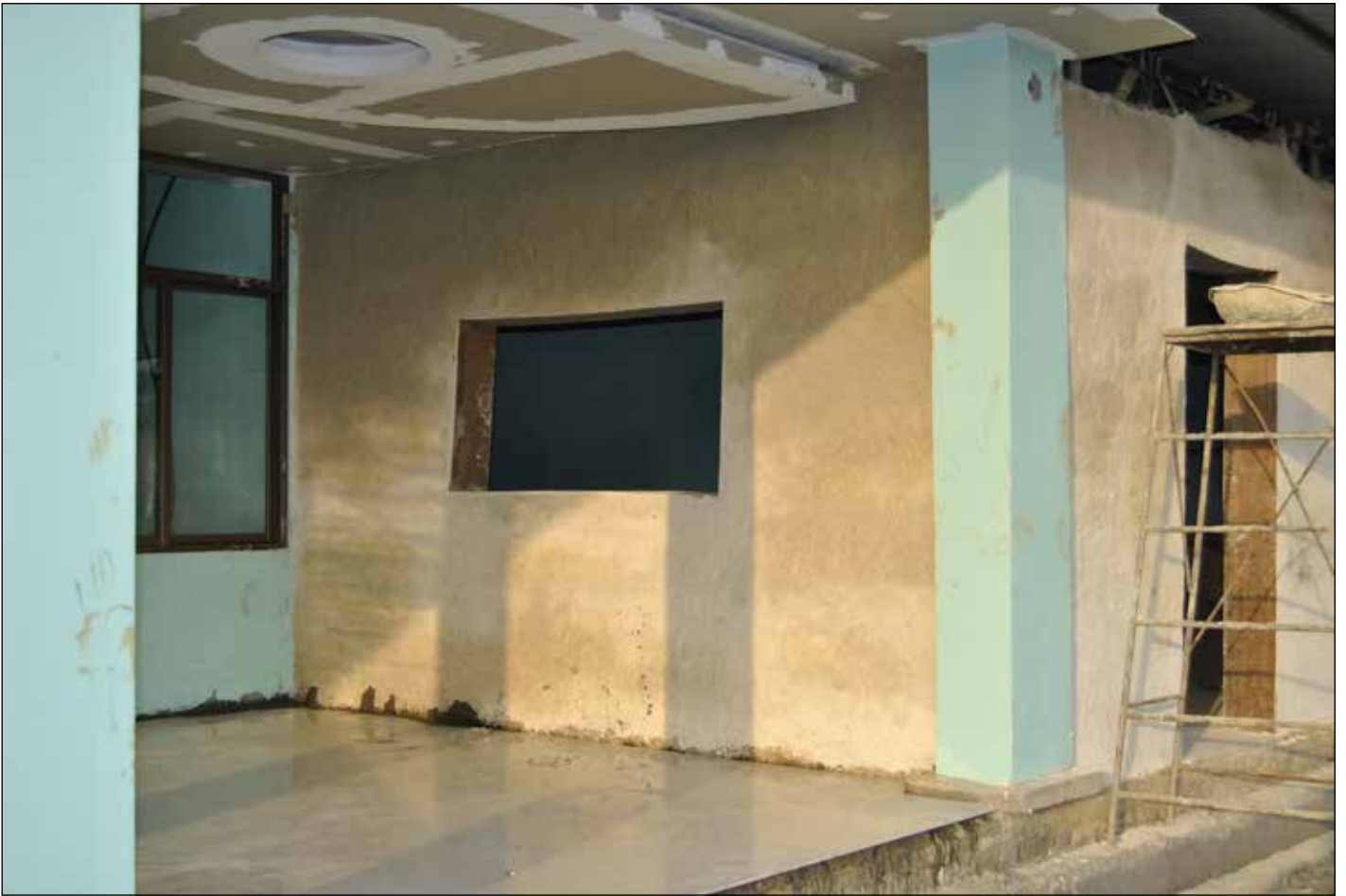
Construction of a Montessori school in Lahan, Nepal, built by SHIV this year.
